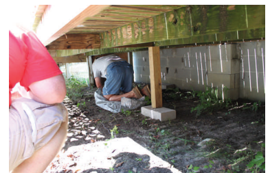
There were no support beams under this porch that was 8' wide X 22' long.
