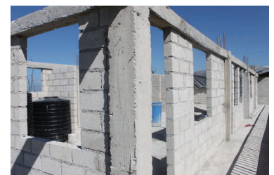
The third floor on the main building that needs a roof and interior walls.
